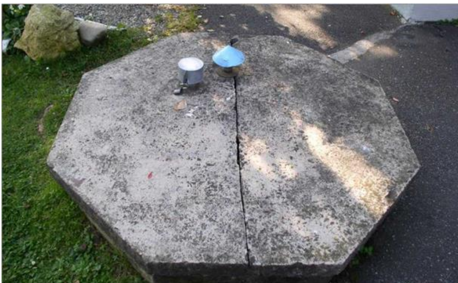
Figure 6: Household well in bad condition, © H. Stadlbauer.
